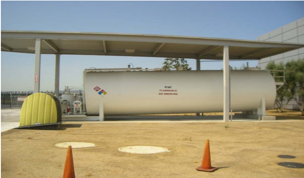
AVBASE ABOVE GROUND FUEL STORAGE TANK
